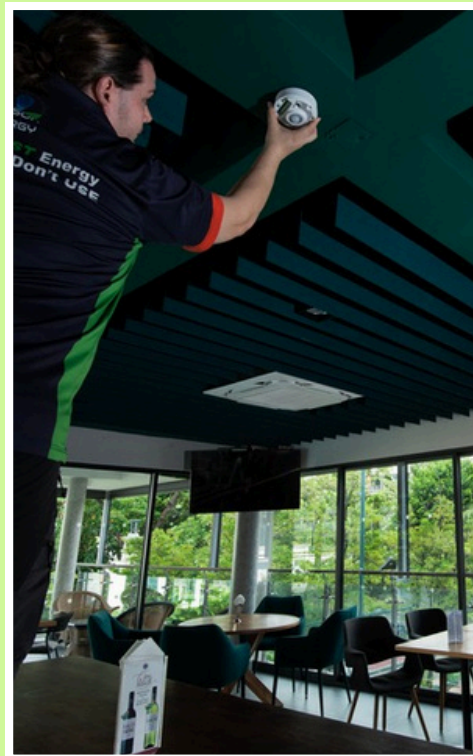
Checking Temperature Sensors
